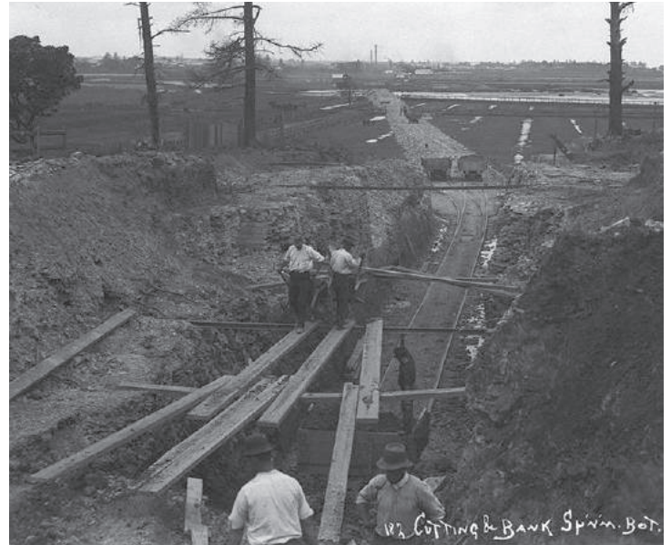
Above: Construction of a cutting (foreground) and embankment (background) for the Botany Line, 1916 - Refer to technical report for source.
