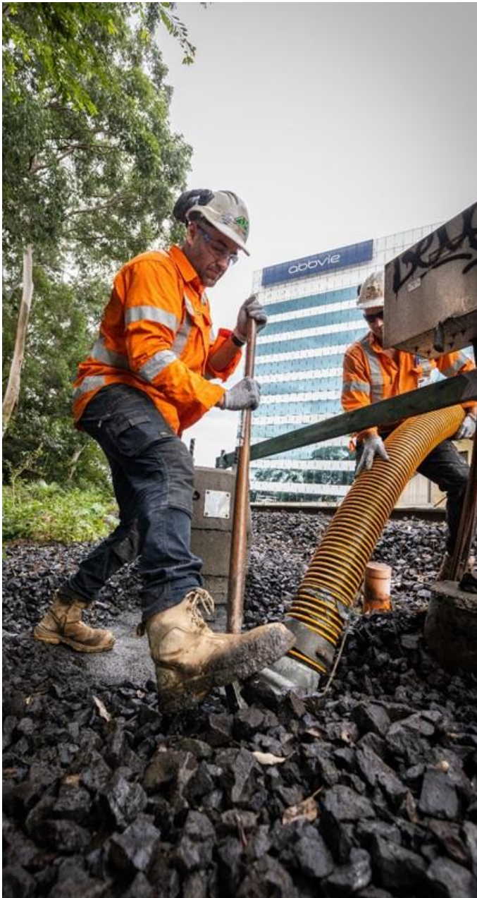
Combined Services Route (CSR) work involving a vacuum truck to help loosen ballast
