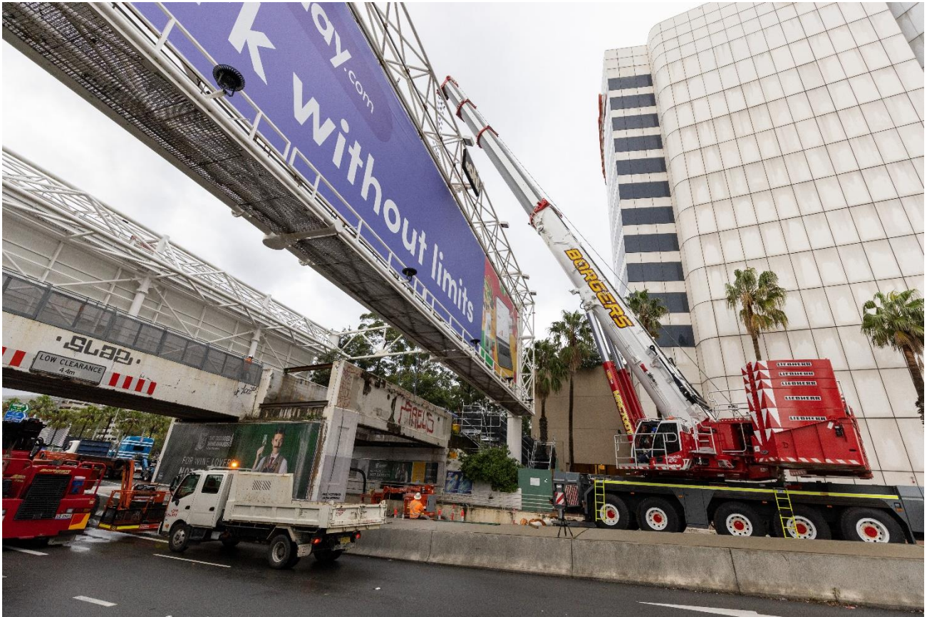
The 650-tonne crane in position at O’Riordan Street during the operation to remove an unused section of bridge.
