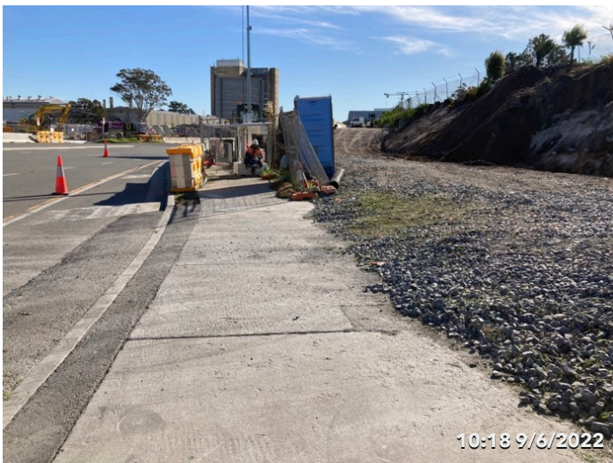
Photo 9 Access at Qantas Drive - stabilised with spill kit available at the entrance.
