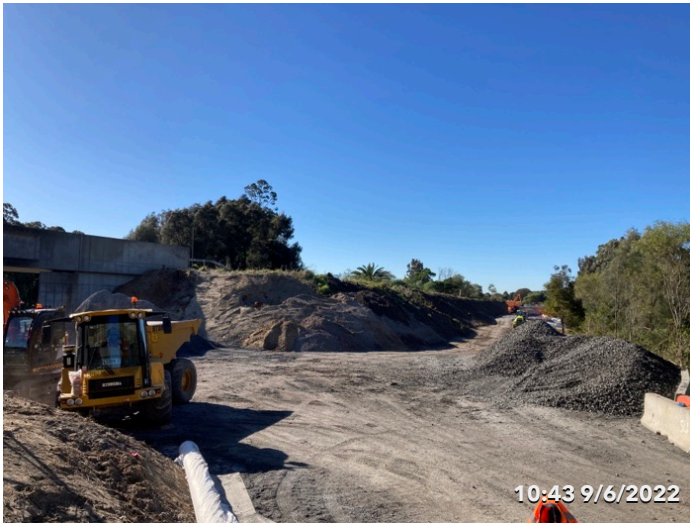
Photo 28 Mill Pond - Stabilised batters on the left and stockpile of ballast on the right
