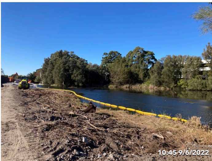
Photo 29 Mill pond - silt curtains installed
