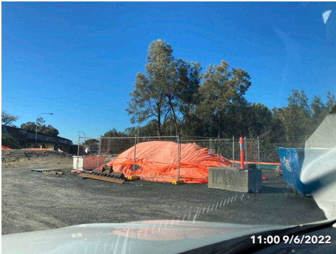
Photo 37 Asbestos containing material stockpile - covered and fenced. Signage also installed.
