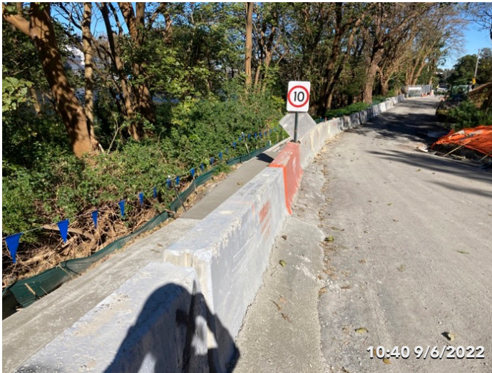
Photo 25 Mill Street - gap between the jersey barriers was also sealed for sediment controls
