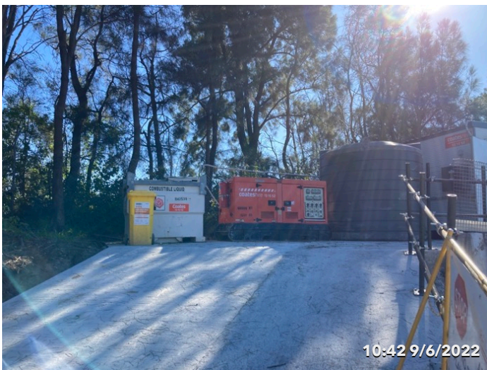
Photo 26 Self bunded fuel tank and generator with spill kits
