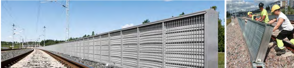
Figure 12 Close-to-rail noise barriers
