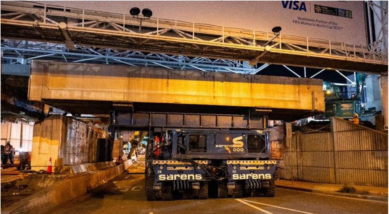
SPMT (self-propelled modular transporter) lowering and removing the existing O’Riordan Street bridge during the five-day planned rail shutdown, before the new bridge was constructed
