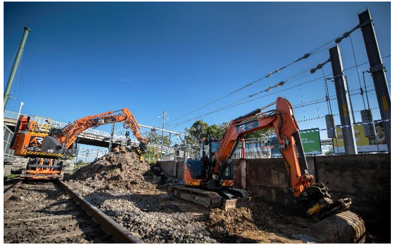
Excavation of existing embankment to make way for new signalling locations at Cabramatta.
