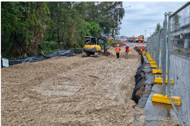
The diverted shared path on the Warwick Farm side of Cabramatta Creek, shown while under construction. This has now been sealed and is open for use.
