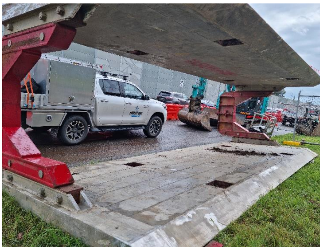
Three large shoring boxes, like the one pictured, will be inserted into the ground between Junction Street and Bridge Street while we install the new stormwater drain. Due to the trench being a deep excavation, these shoring boxes are required to support the sides. As we move up the road, these get moved through the trench to where they are needed.
