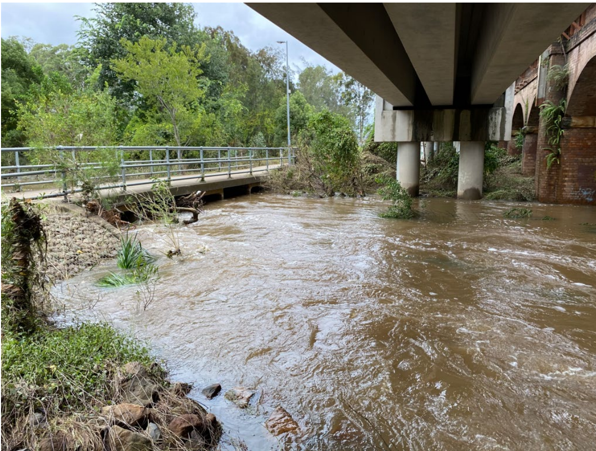
Cabramatta Creek culvert crossing looking from upstream after flooding rain event, March 2022
