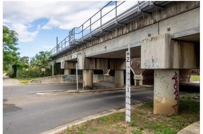
The existing rail bridge at Sussex Street, where it joins Broomfield Street.
