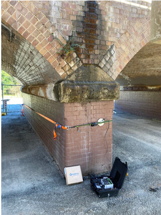
Above: Monitoring setup of the heritage bridge that carries Sydney Trains. The device was firmly strapped to the pylon during monitoring.
