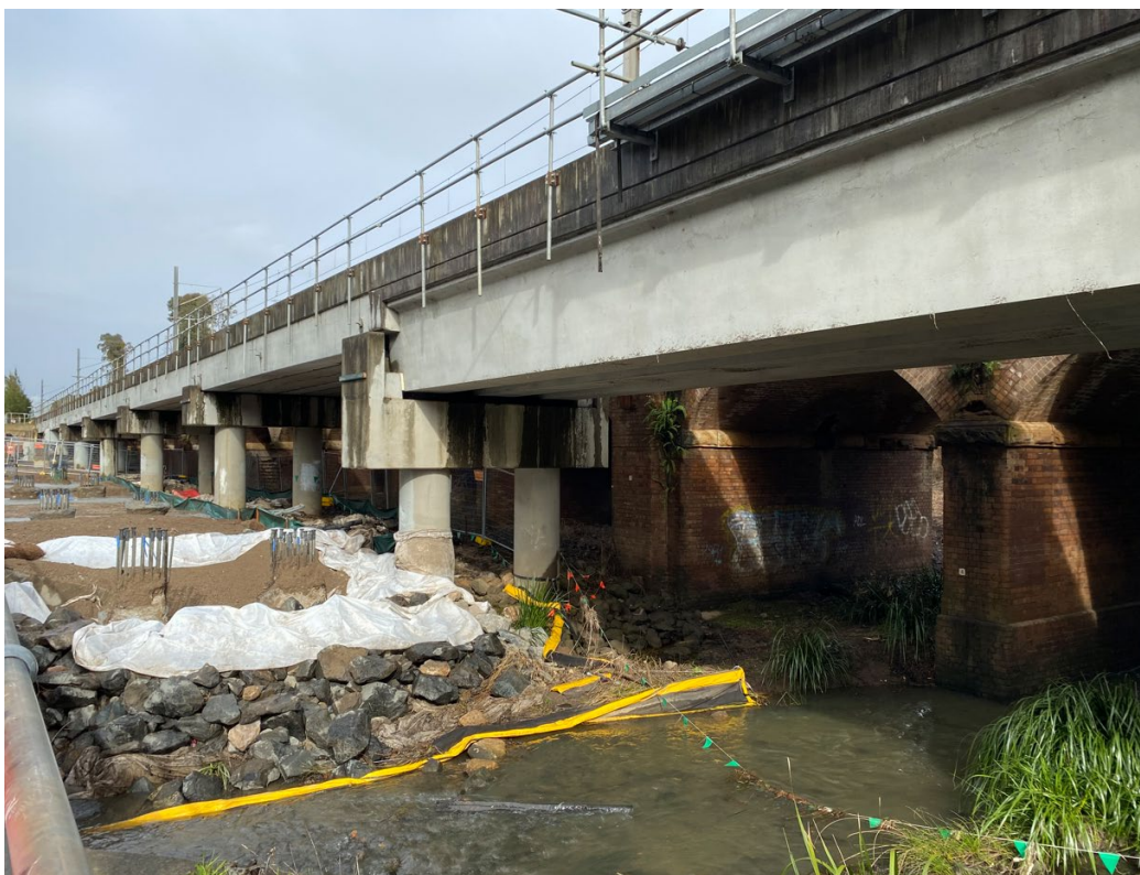
Above: Piling pad establishment at Cabramatta Creek during the end of July
