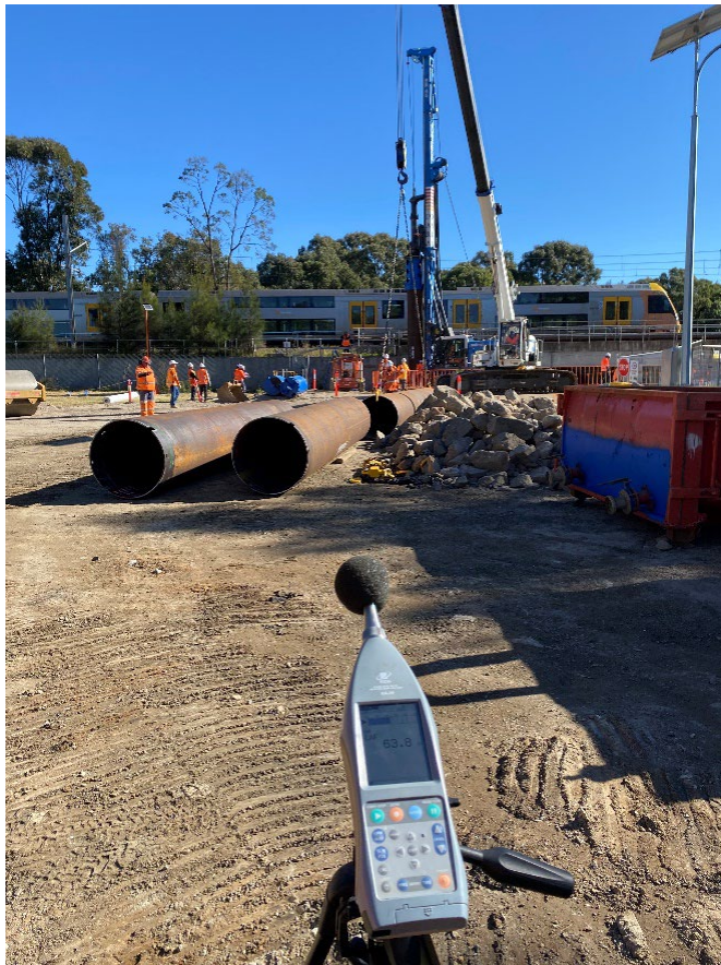
Above: Test monitoring of piling rig on the 9 th June 2022, weeks prior to works near the sensitive receivers at Sussex Street and along Broomfield Street.
