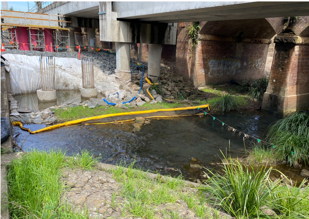
Above: Progression of piling and bridge works at Cabramatta Creek during September
