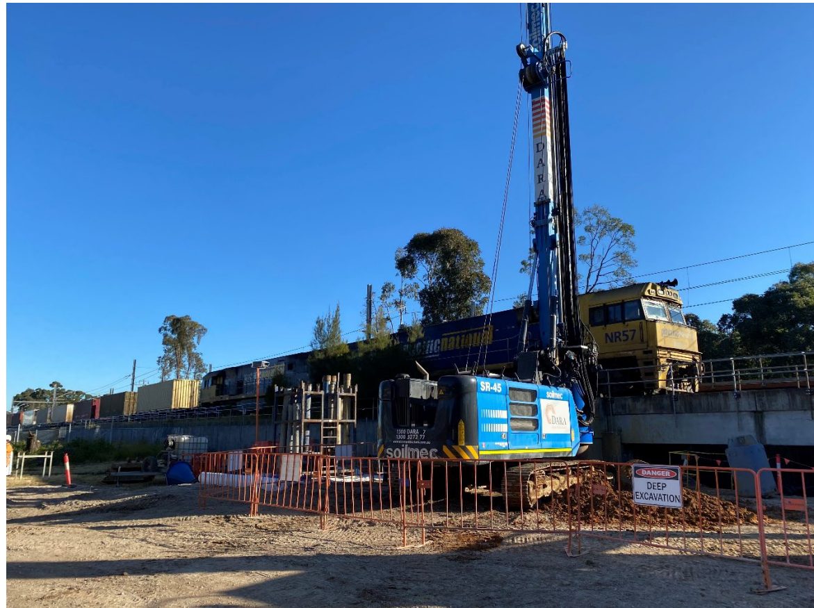
Above: Typical piling activity during monitoring in June. Piling progressed northward over the course of the month.
