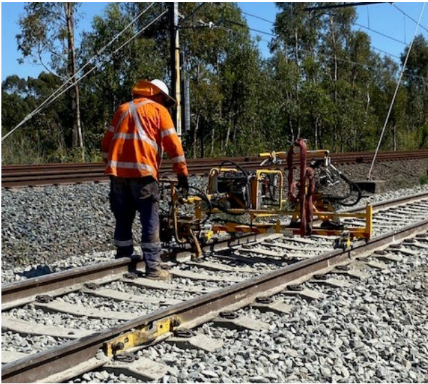
This machine clamps clips to the rail, to keep it fixed in place
