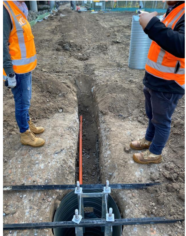
Getting ready to install the street light pole for the new pedestrian and cycle path
