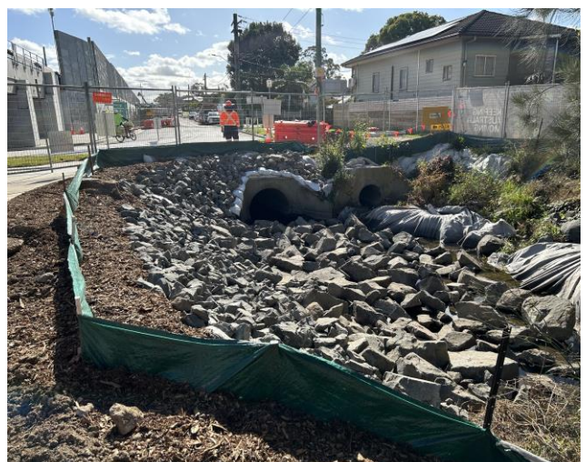
Scour rock installation at the stormwater outlets near Sussex St, Cabramatta. The area is also surrounded by green silt fencing.
