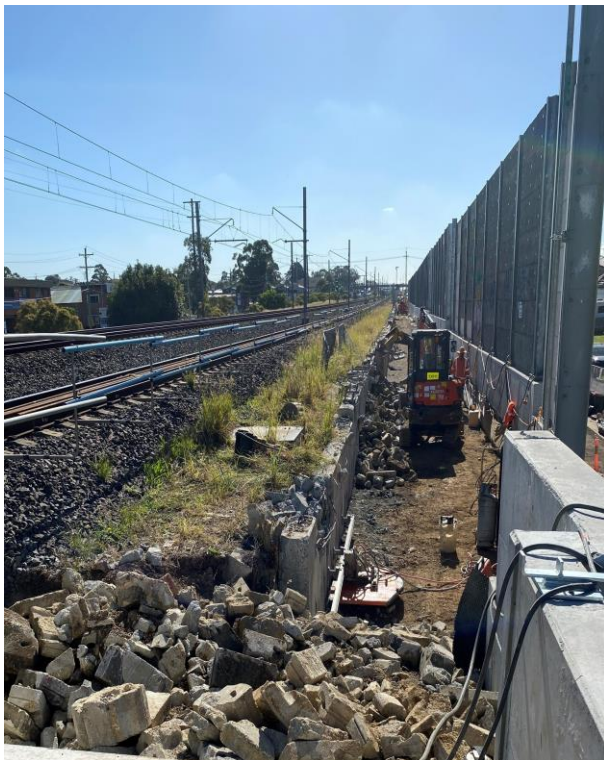
Removing the original Broomfield Street noise wall to make space for the new track
