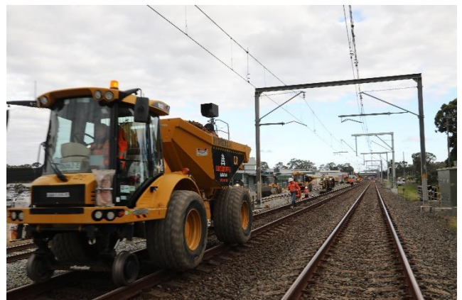
Truck delivering ballast to be laid on the track during 54-hour shutdown.
