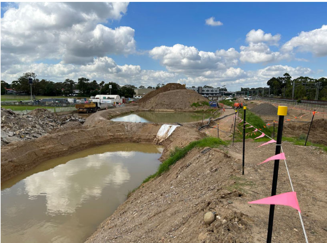
Above: Storage of site water within treatment basins at Jacqui Osmond Reserve following rainfall in February 2023.
