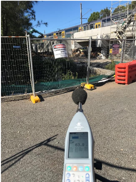
Above: Attended monitoring at 10 Sussex St, Cabramatta during WE32 possession in February 2023.
