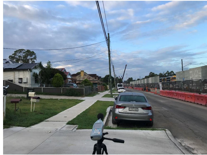
Above: Monitoring at 150 Broomfield St during OOH girder lift on the 3 rd of March 2023.
