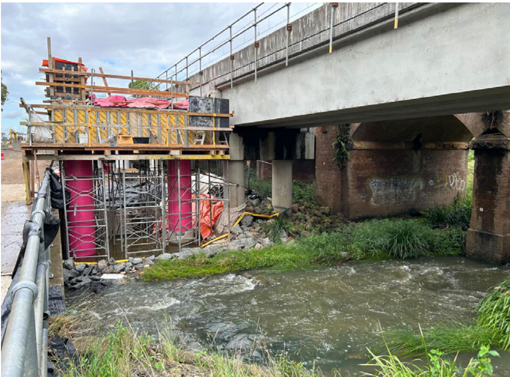
Above: Progression of bridge works at Cabramatta Creek following a minor rainfall event in February 2023.
