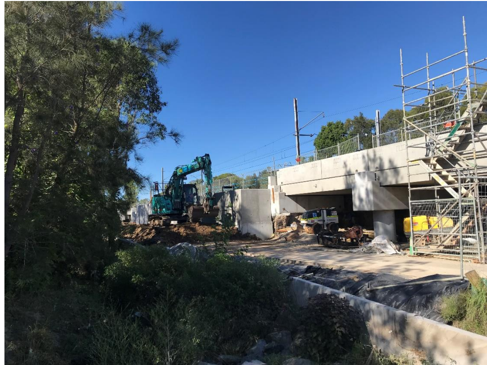
Above: A closer view of the works monitored at 10 Sussex St (RW10 backfill) during WE32 possession in February 2023.
