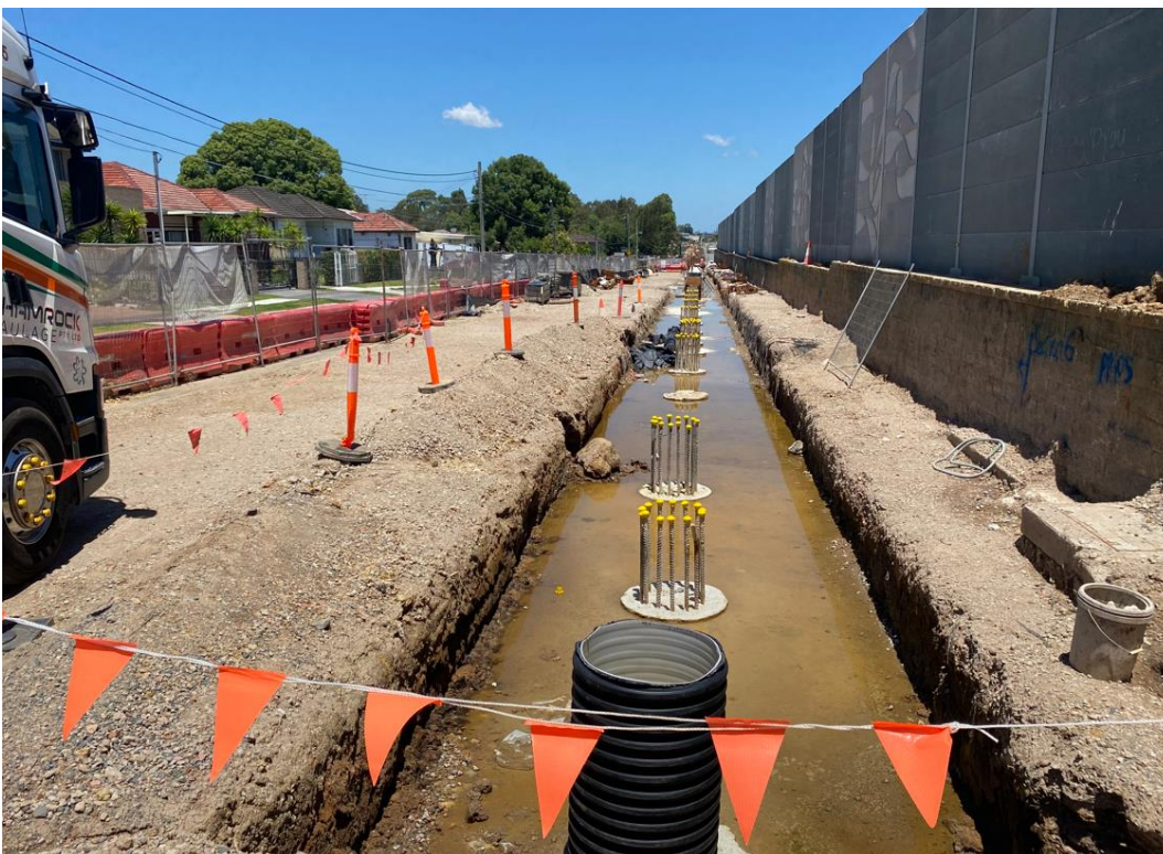
Above: Excavations holding water following a minor rainfall event in January 2023
