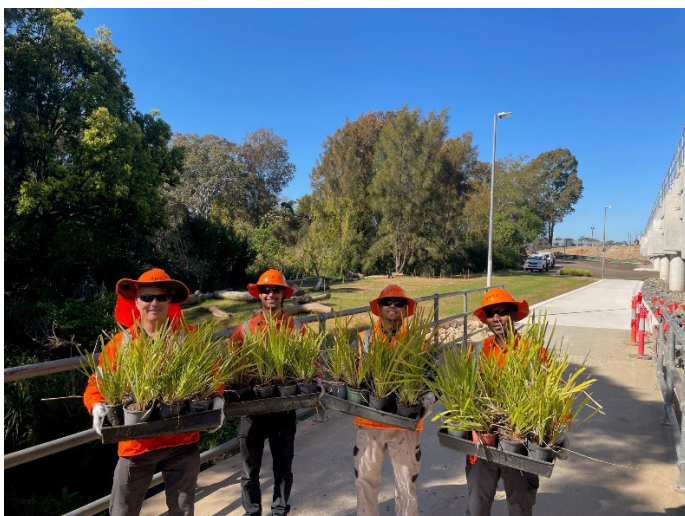
ARTC project team helping with landscaping the area near Cabramatta Creek Bridge
