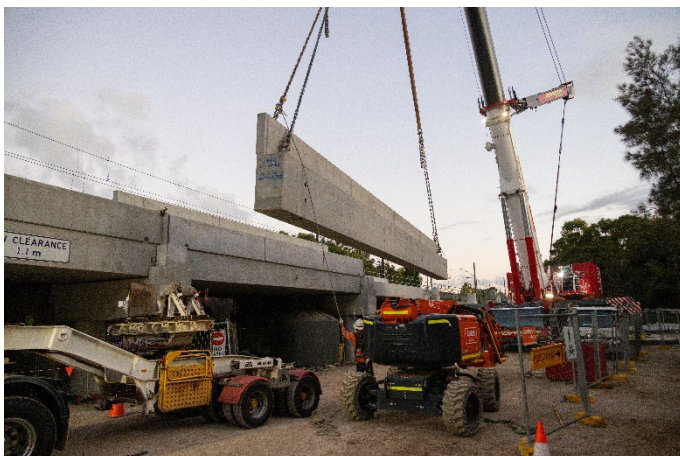
Lifting concrete beam into place for the new Cabramatta Creek bridge duplication
