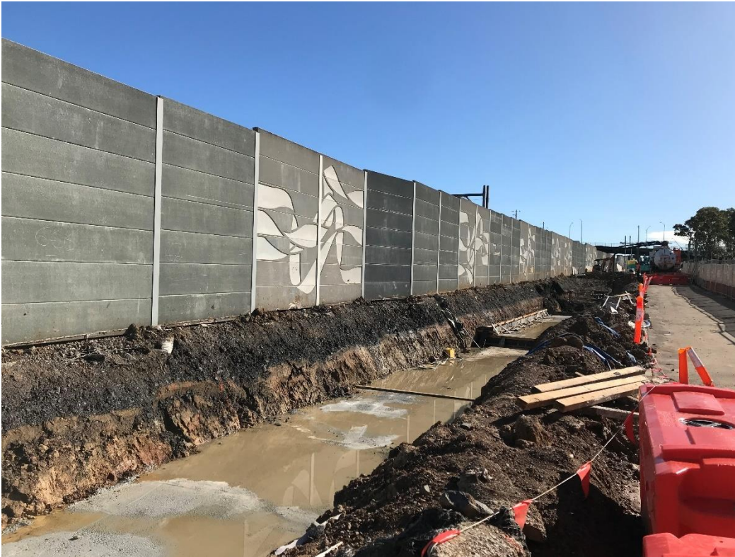
Above: Excavations holding water following a minor rainfall event in May 2023
